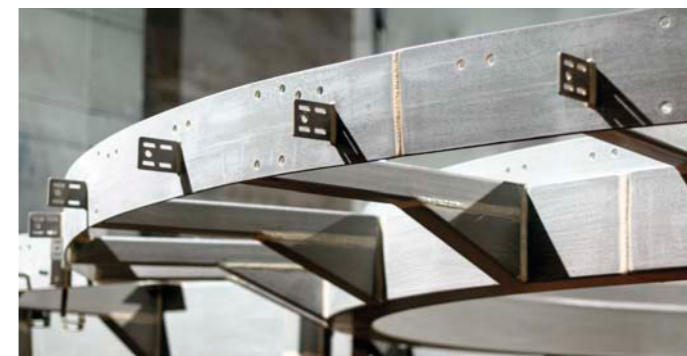
Before spray painting, all the joints, the necessary edges and elements, as well as confined areas were prepared manually (with the use of the stripe coating technique), so as to guarantee full paint penetration in such places.
