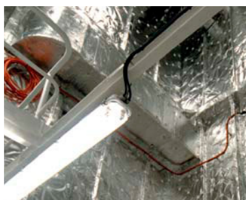
Energy-consuming and fire-resistant insulation in the funnel casing.
